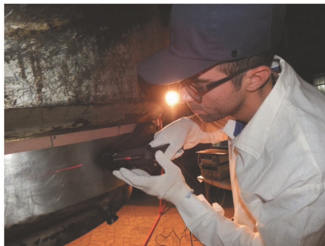
Figure 1. Manual CPD measurements of the input and output pipes in steam generator at the places where they were welded to the corresponding collectors.
